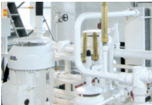
Detail of piping system
